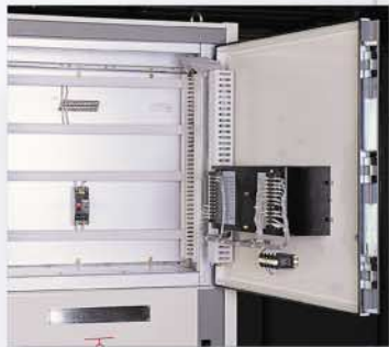
Low Voltage Compartment
